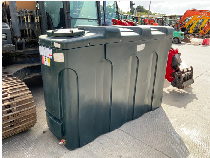
2000LTR BUNDED HEATING OIL TANK
