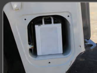
Battery Access Panel
